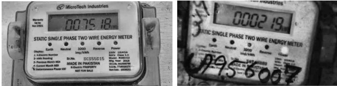
Figure 1. K-Electric electricity meters.
