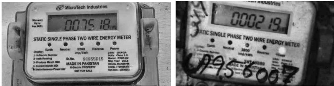
Figure 1. K-Electric electricity meters.
